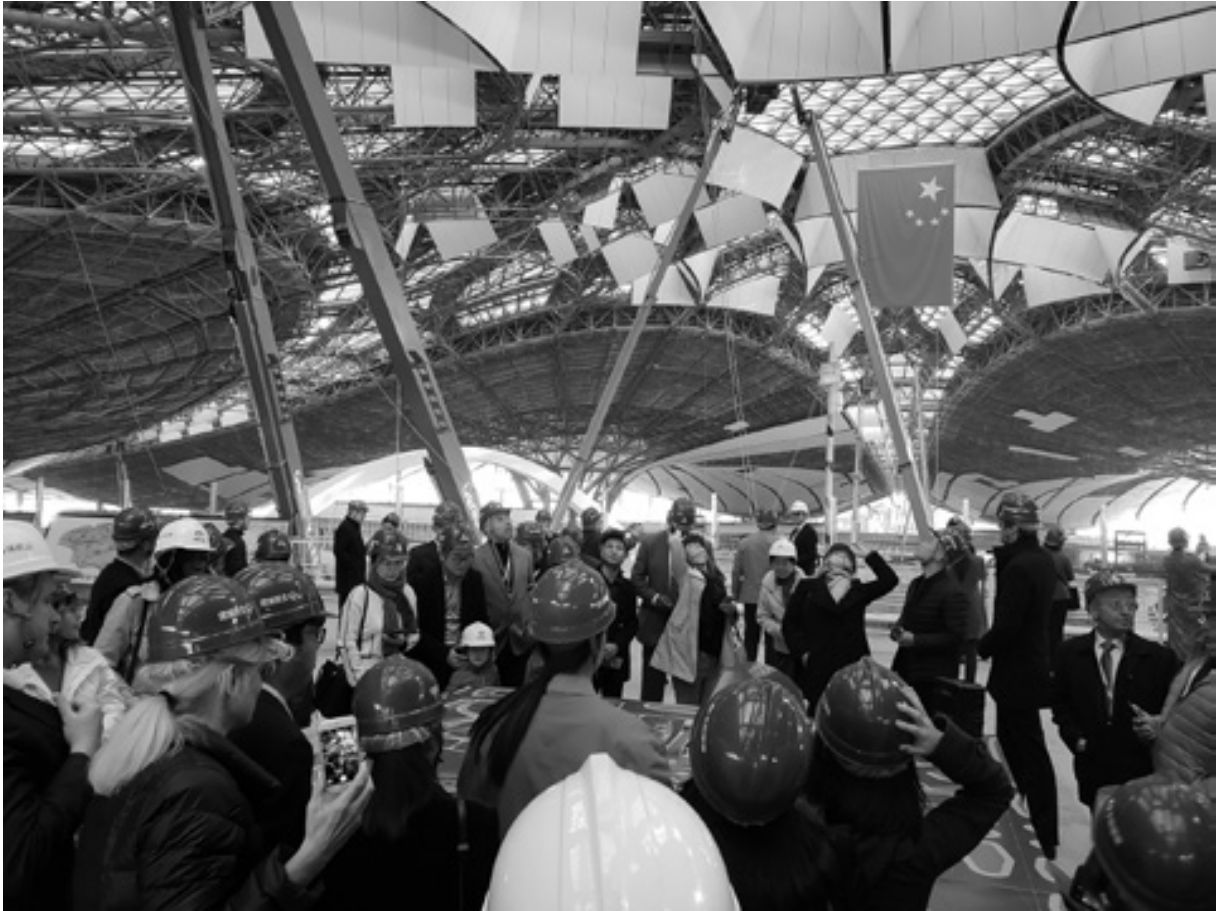
Figure 10.1. Aviation professionals visit the construction site at Beijing's Daxing International Airport. (Photograph by Max Hirsh.)
